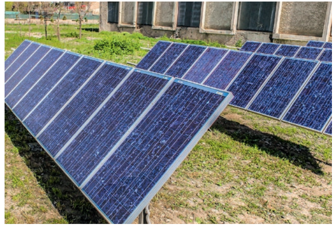
Renewable energy systems were handed over to the Afghan energy supplier | © GIZ
